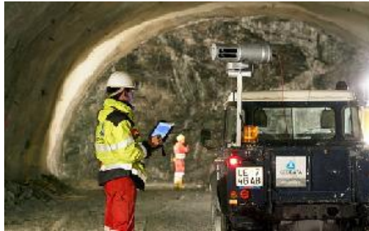
Laser scanner on a vehicle in the heading area (Tunnel Kirchdorf, Austria)
