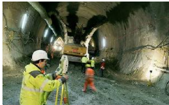
Heading control of side-wall drifts during construction (Lainzer Tunnel lot 31, Vienna, Austria)
