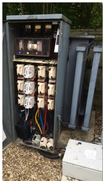
Real 500 kVA Transformer
