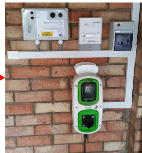
ROLEC* charging point + EA Technology Intelligent Control Box
